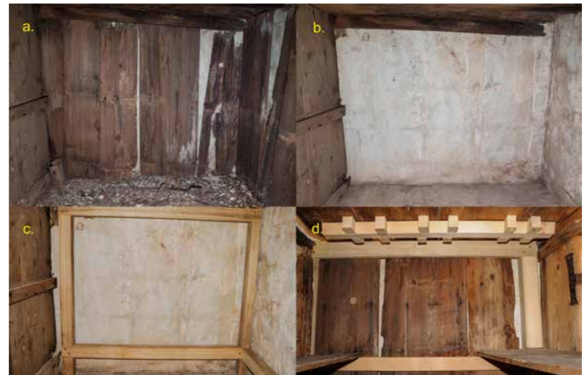
Figure 8a – 8d Series of photos from the inside of the parament cabinet: Figure 8a Right-hand compartment of the parament cabinet before cleaning (2014); Figure 8b after cleaning and dismantling of several boards; Figure 8c insertion of an auxiliary structure made of Accoya wood; 8d the old boards are reattached to the scaffold; a ridge strip was installed to stabilise the tabletop (2016).
